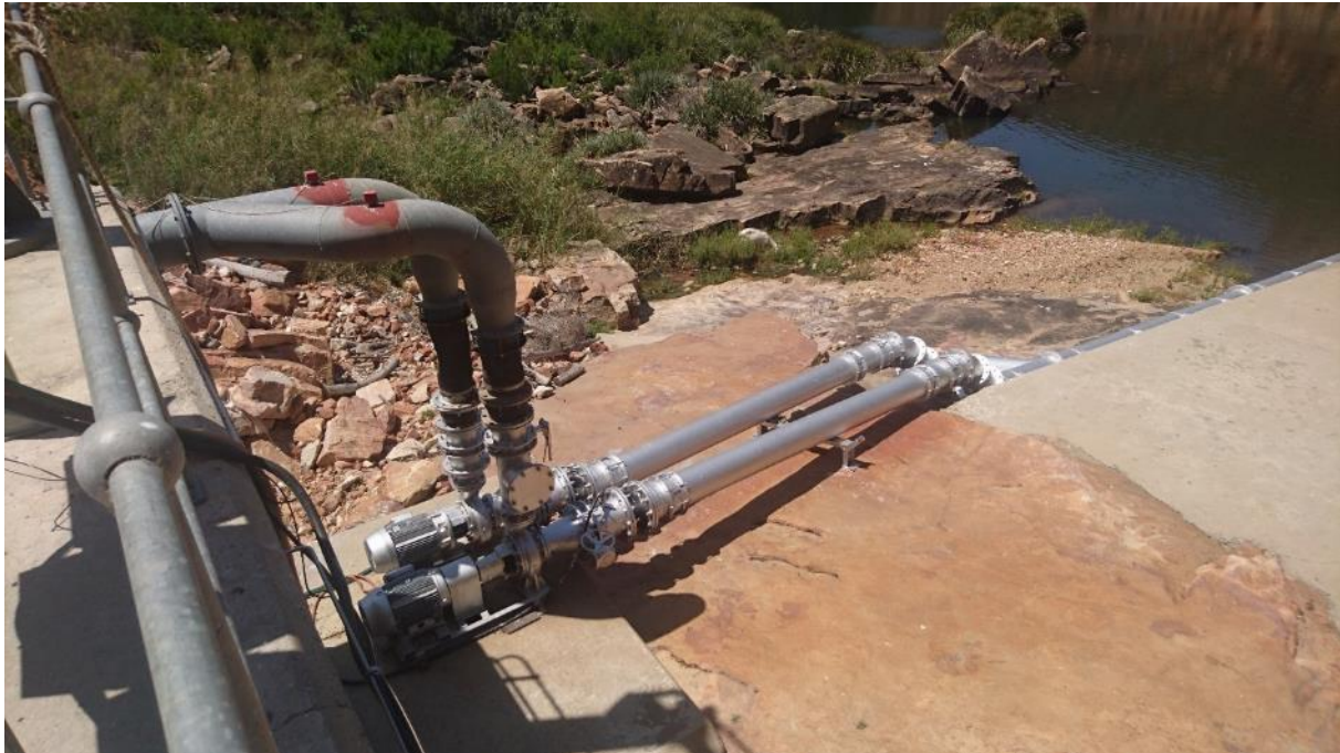
Figure 3.7 | Pumping system installed at Bulshoek Weir to recover leakage
