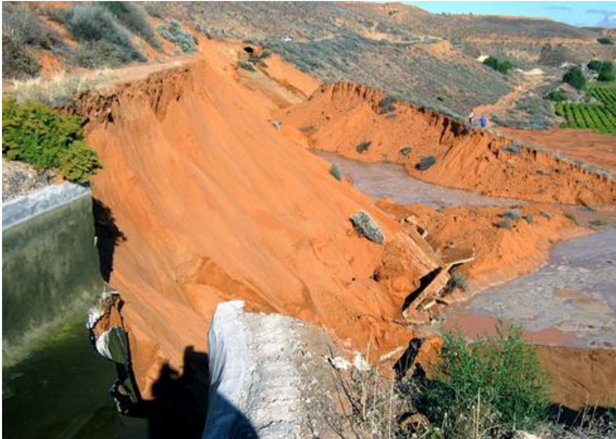
Figure 3.11 | Lower Olifants Canal break in 2015 (IOL, 2015)
